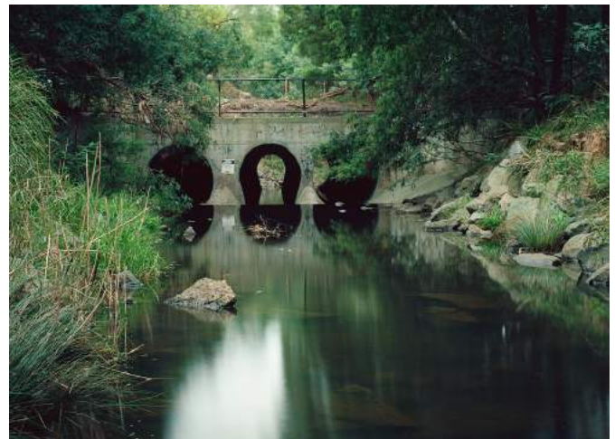
Figure 33. Urban Stormwater Drainage
