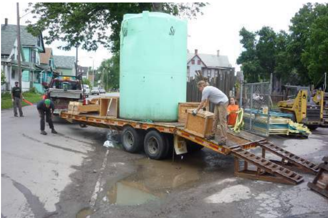
Figure 40. Rainwater Collection Tank
