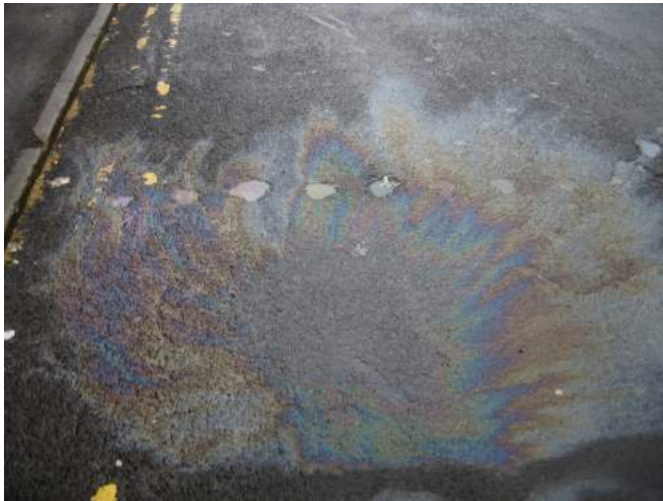
Figure 32. Oil on Pavement
